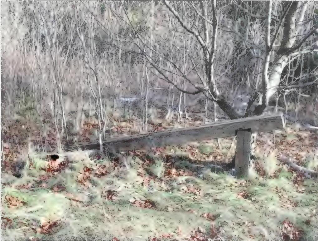
Figure 3.57. View looking east at collapsed wood guardrail, Battery Kingman. Across from both gun emplacements, a series of wood guardrails are installed along the eastern edge of the unpaved road. The guardrails are in fair to poor condition (Olmsted Center, January 2009).
